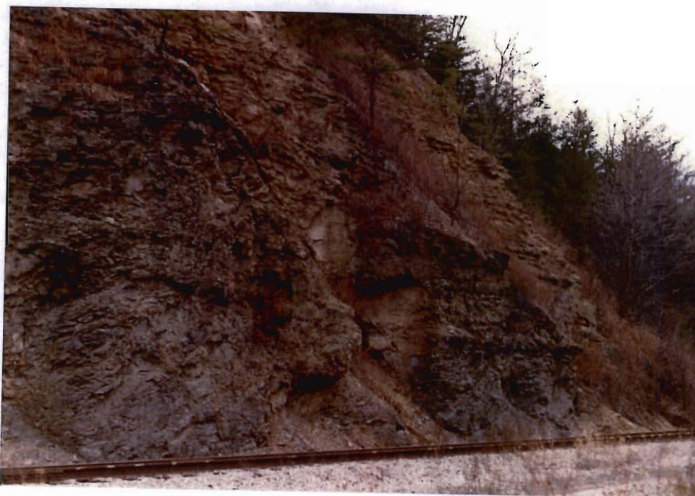
Figure 14. Parallel fractures at Field Station 55.
